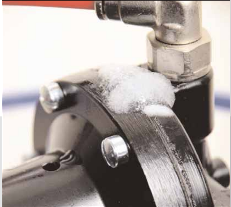
Figure 5. Leakage can be from any joint and is easily shown by spotleak.
